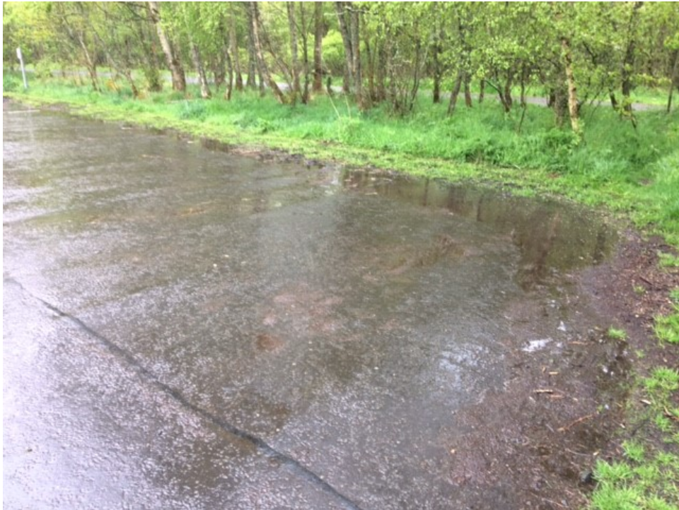
Figure 3 Additional work on drainage and bay delineation required
