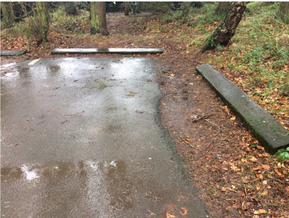
Figure 2 Damaged edging replacements and full bay lining required
